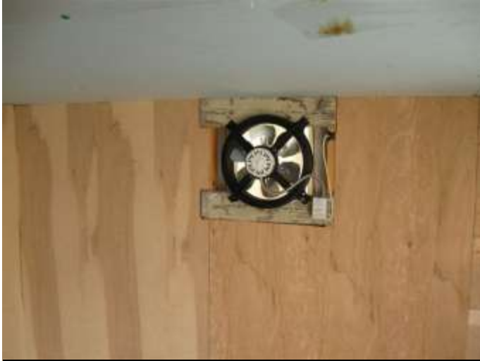
Meg's Place ventilation system
