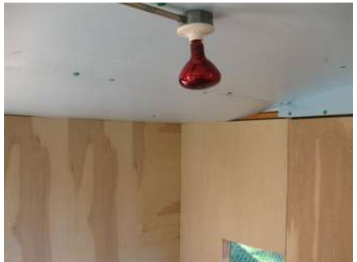
Meg's Place heating element
